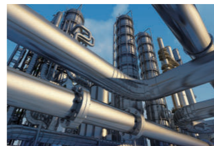
Gas Cleaning Desulphurisation
